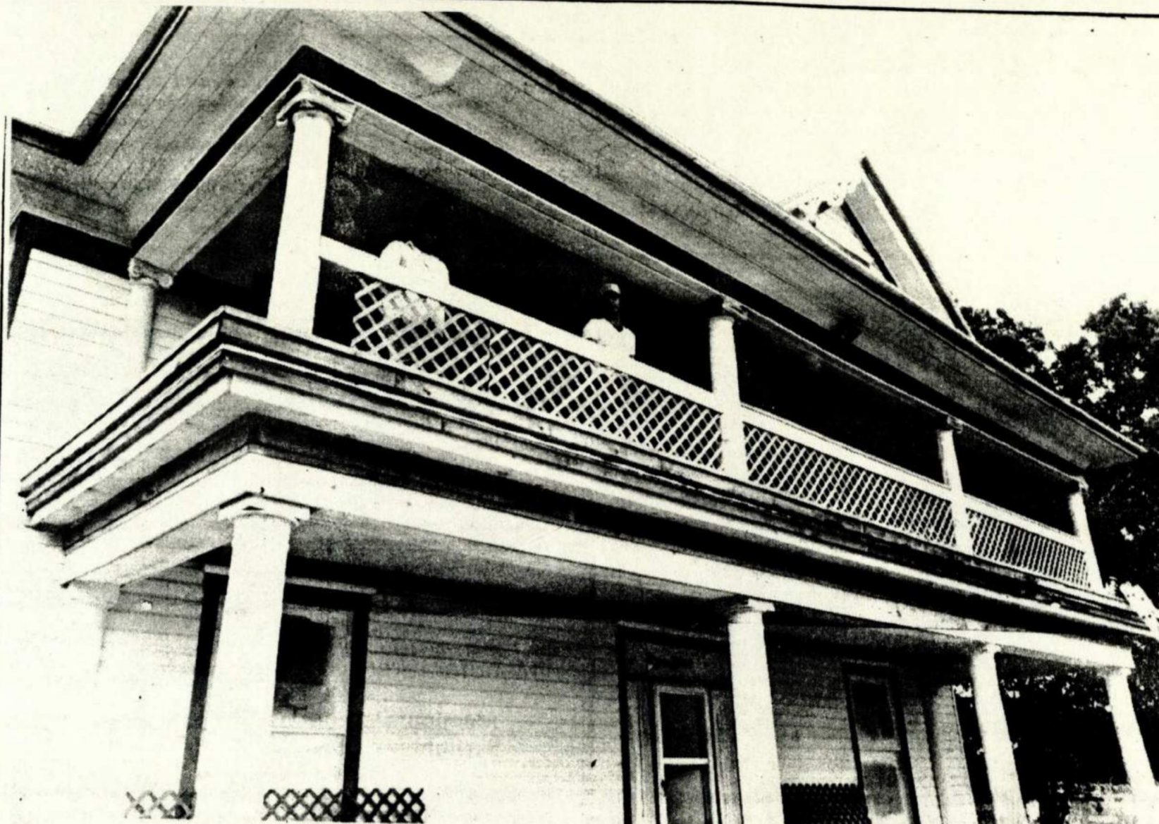
As part of the renovation effort, the balcony railing on the Back home on Smith Street is placed by homeowner Paul Round-
