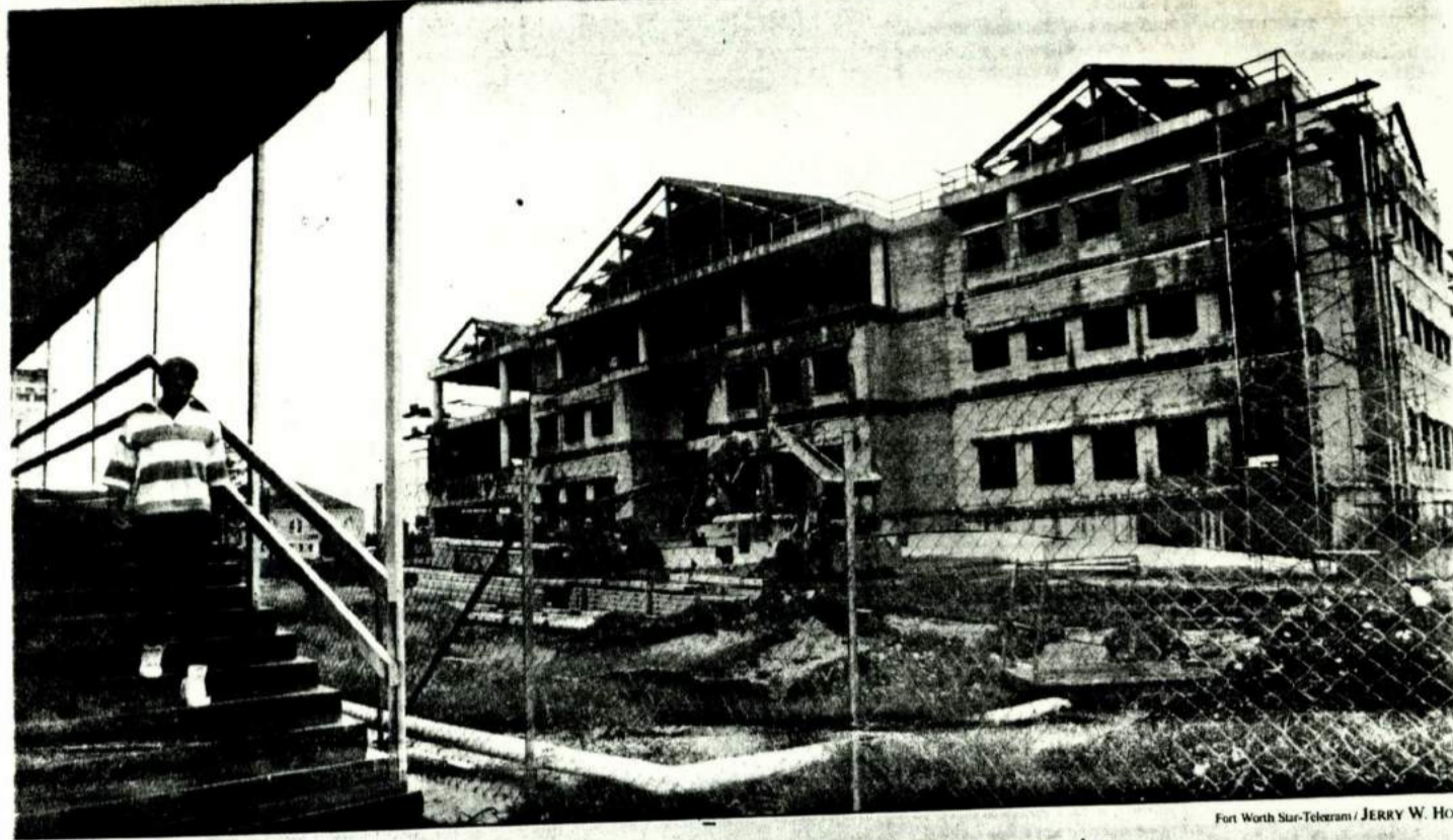
Student Jeff Buck walks near the new Texas Wesleyan College library under construction
